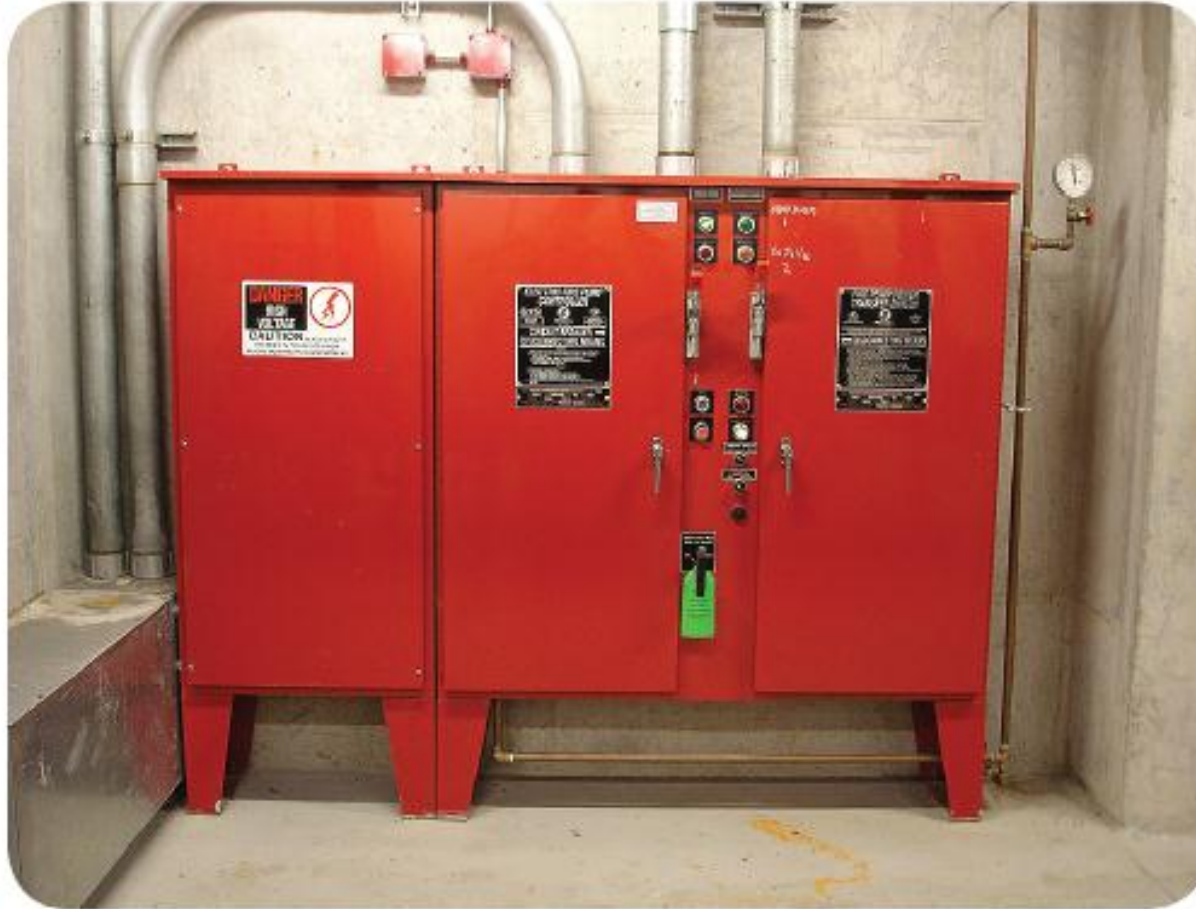
Listed fire pump controller and power transfer switch.
