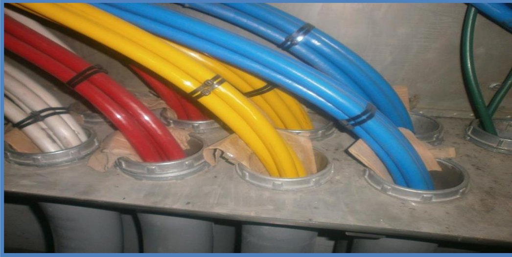
Improper cable grouping
