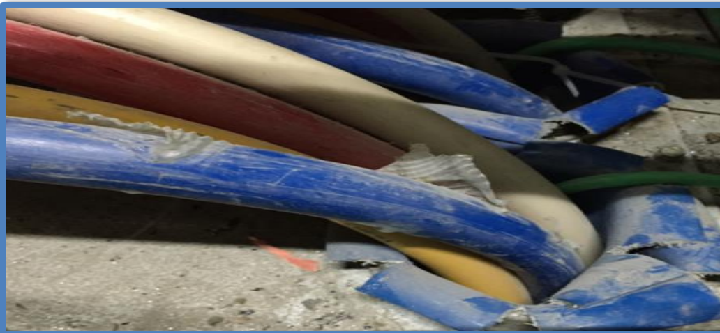
Cable damage during cable pulling and installation
