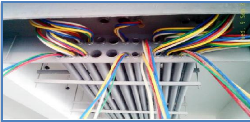
Overbending of cable on pull boxes
